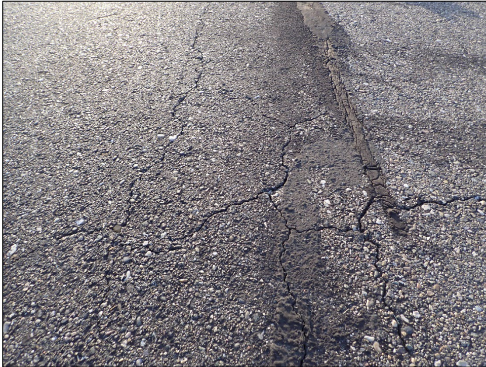
TW-04-05: Alligator Cracking
