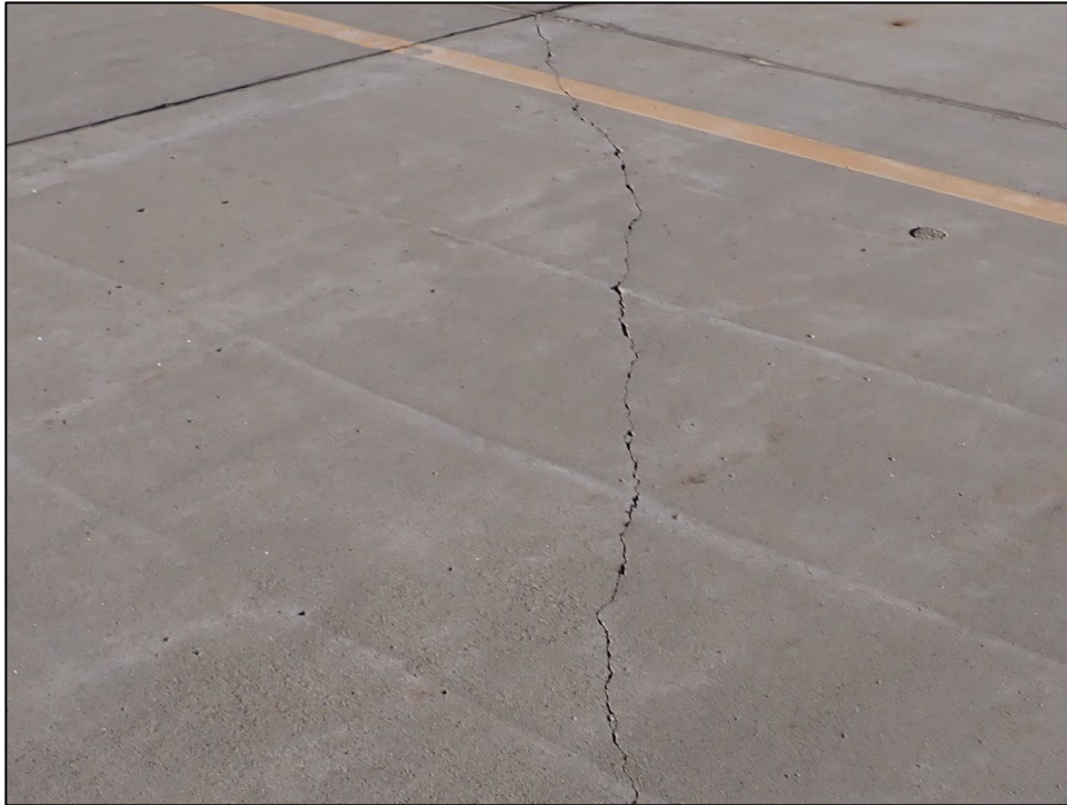
AP-06-03: LTD Cracking
