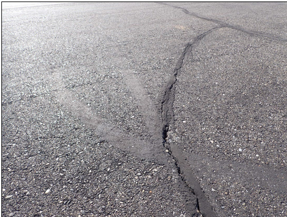
TW-01-07: L&T Cracking
