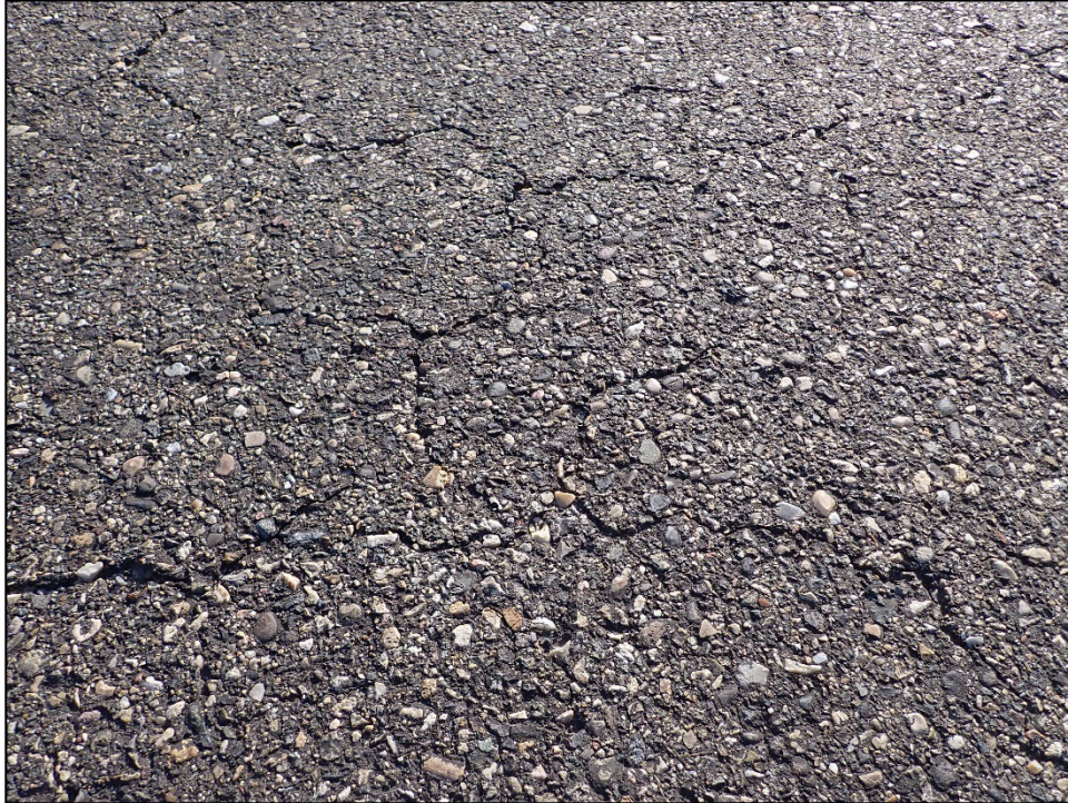
AP-03A-01: Alligator Cracking
