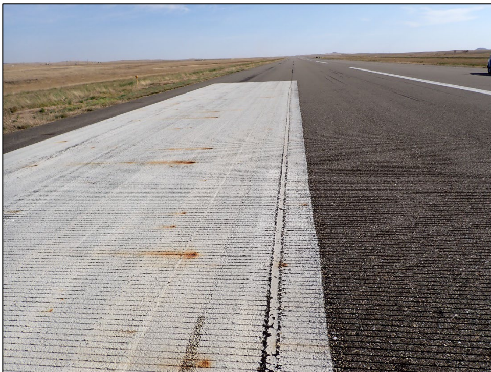
RW13-01-18: L&T Cracking
