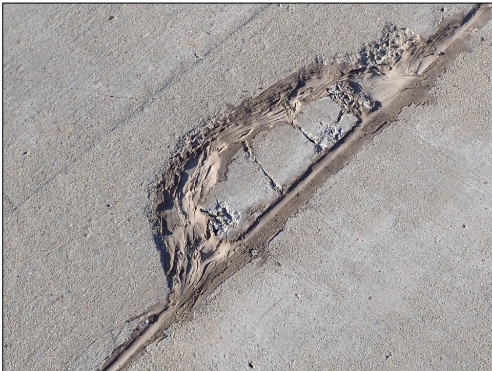
AP-06-03: Joint Spalling
